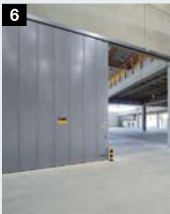
6 Fire sliding doors
